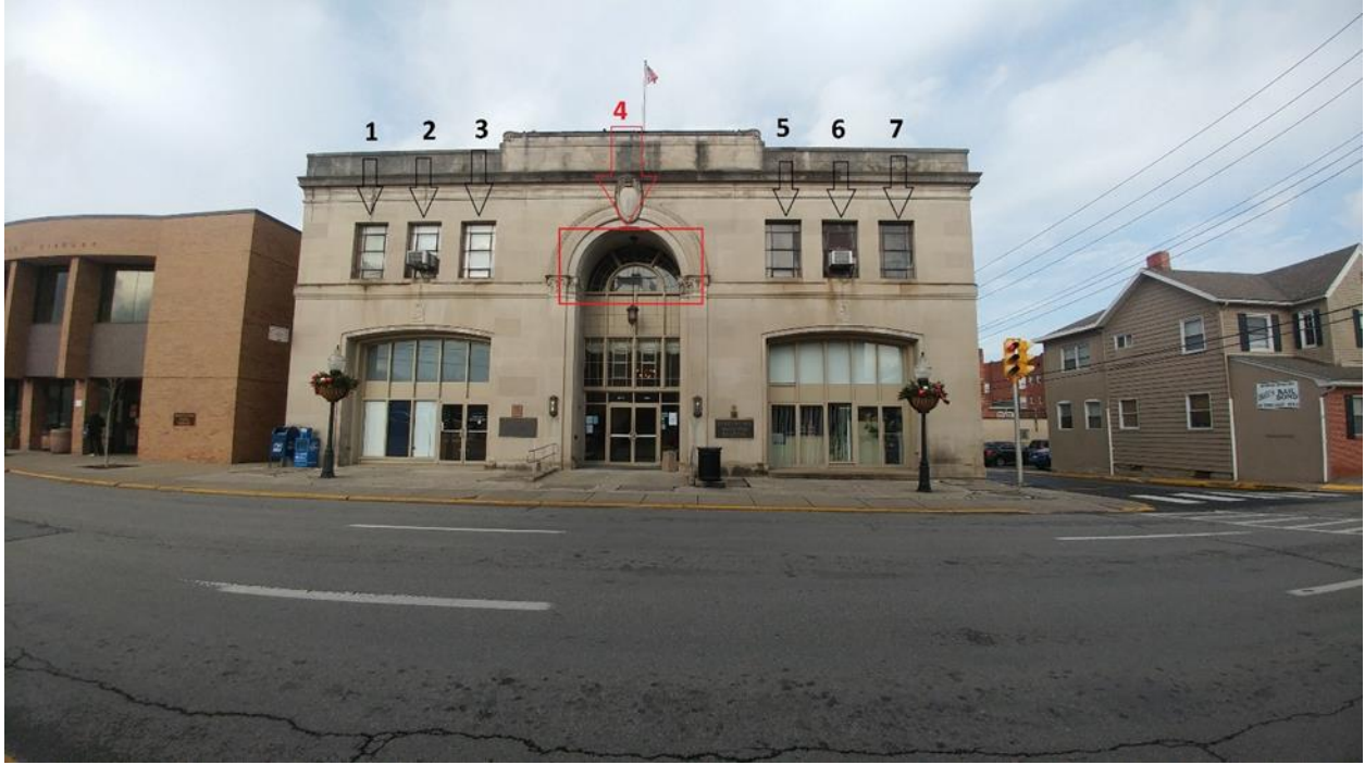
Figure 3: Windows that need to be restored/replaced.
