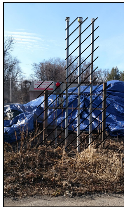
PHOTO 2: VENT PIPING AND PIPING STAND
