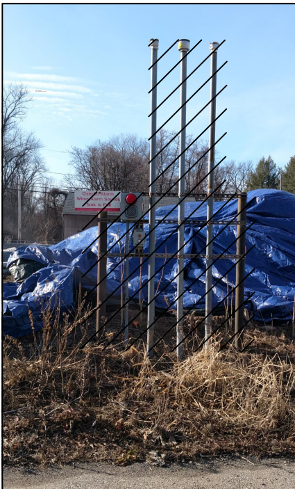
PHOTO 2: VENT PIPING AND PIPING STAND
