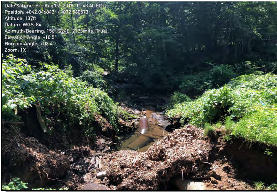
Photo 2: View of downstream of collapsed drainage pipe (JMM photo taken 8/2/19); facing southeasterly
