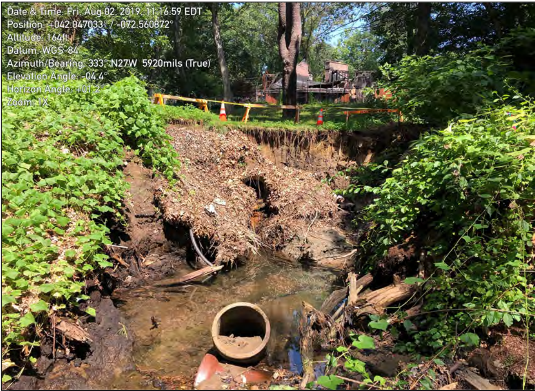
Photo 1: View of collapsed drainage pipe within the western part of JMM Study Area (JMM photo taken 8/2/19); facing northwesterly
